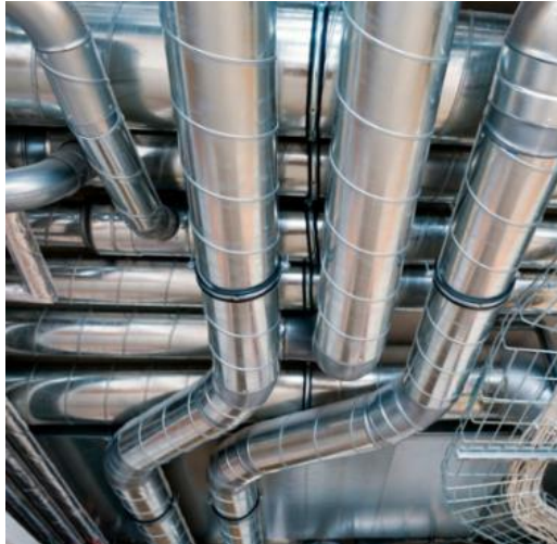
Figure 2 – Air ducts made of metal
