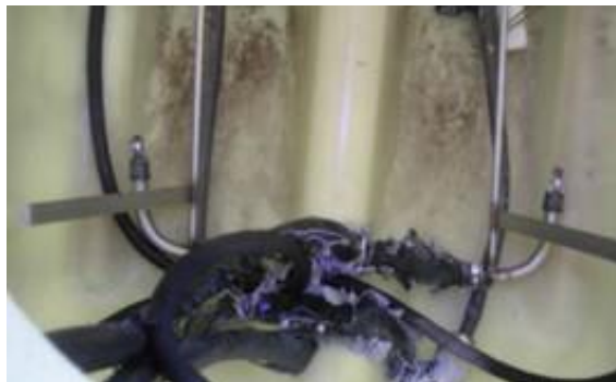
Fig. 2. Tubes and hoses after testing cheap generics
