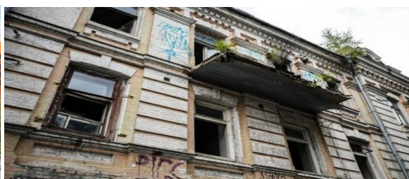
Fig. 2 A building that needs renovation
