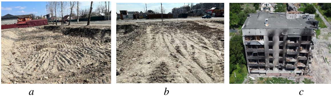
Fig. 1 Site of works: a – section 40 m; b – 12 m section – road between houses; c - section 43 m - with a building that needs to be dismantled.
