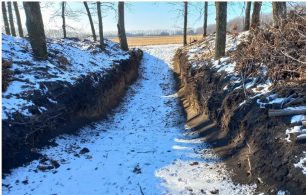
Figure. 1. A trench in the windbreak to shelter heavy equipment (Photo: Petro Ternopilskyi)
