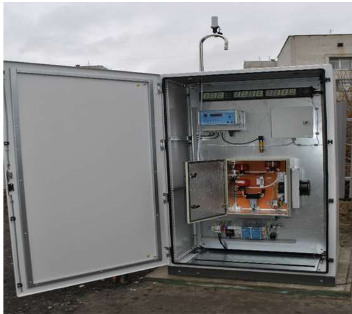
Figure 3.7 – Stationary post of the automated atmospheric air monitoring system of the Kiev Regional State Administration 20
