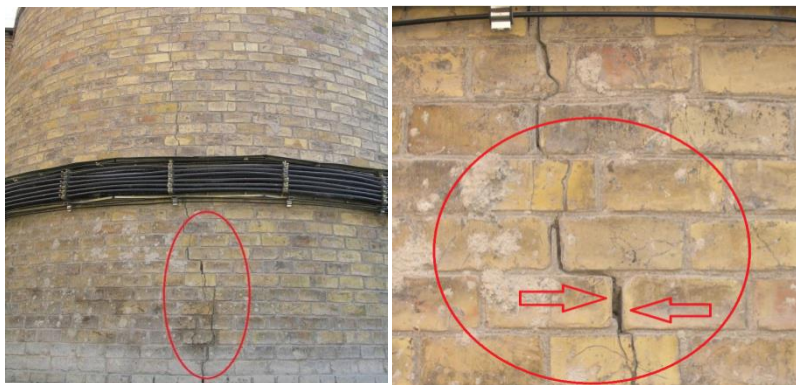
Photo 1 – 2. Cracks in the seams of the brickwork of the stack.
